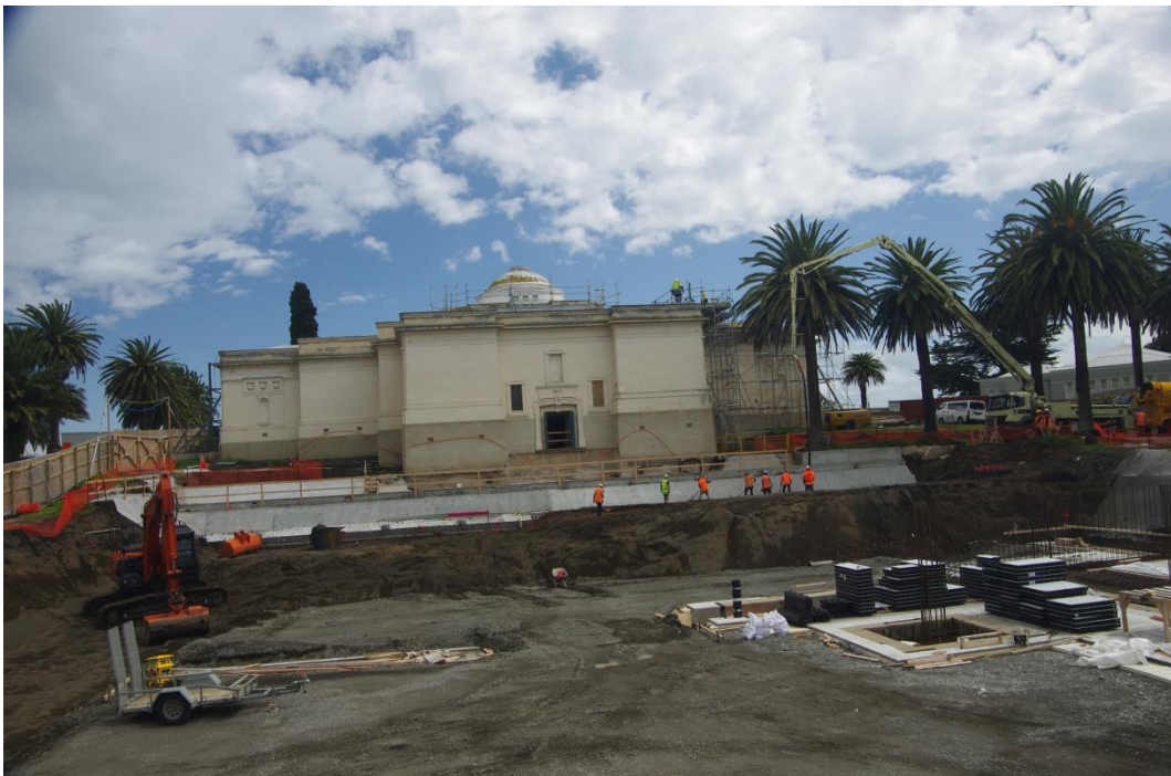
Figure 5: View showing the scale of the basement excavation at the SAG for the new building. Concrete is being poured for the beams across the back of the original SAG building. Cottage 1 (see report Section 3.0) was located to the right of the concrete workers in the image but the archaeologists were stood down at the time the photograph was taken for safety reasons as the concrete pump extended over their work area at the cottage site (Archaeology North Ltd.).
