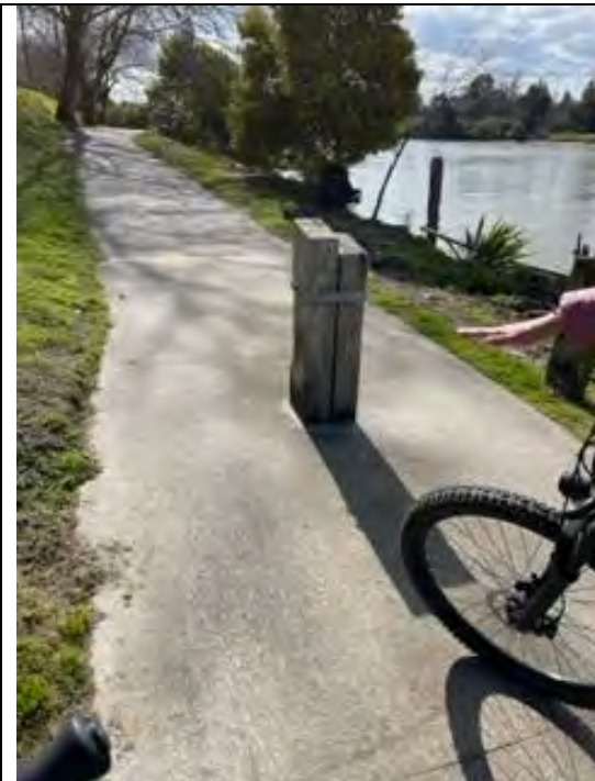
Old bollards. These need replacing over time.
