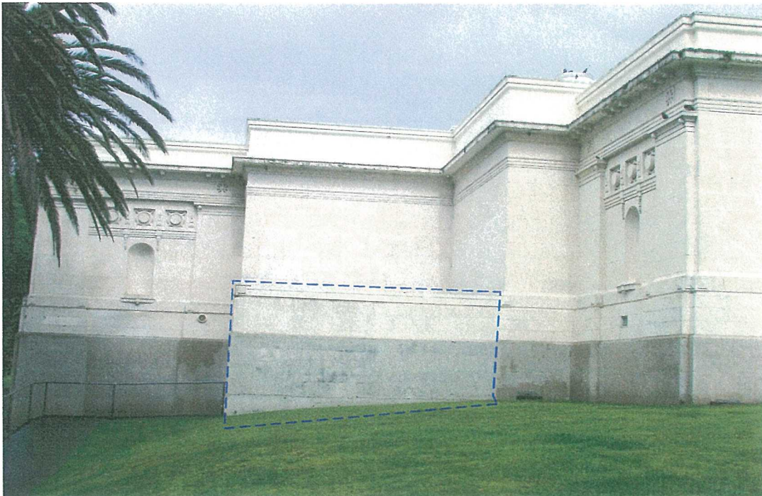
Photograph 4 : View of the gallery back wall to be replaced where trenching will be required during the refurbishment.
