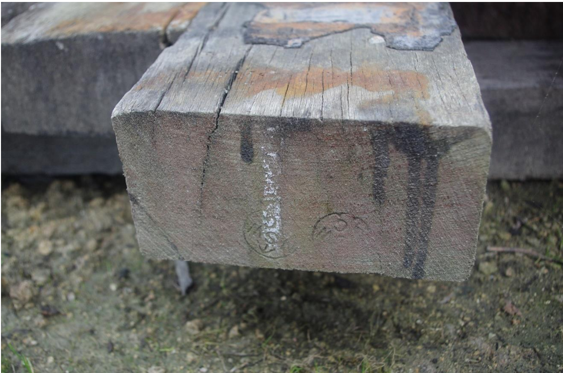
Figure 60: Stock pile, deck joist. NSW Government mark GG (Grey Gum), inspector identified by rim markings
