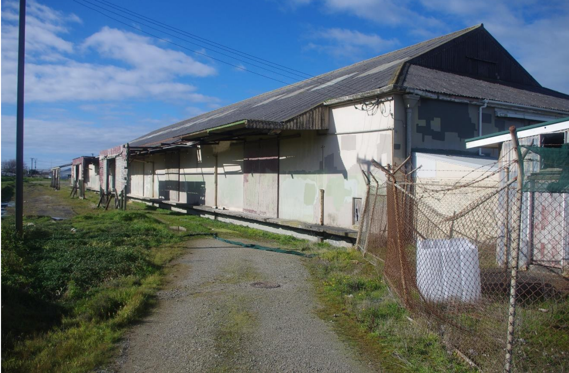
Figure 93: Victory shed with awning and railway siding along northern wall, looking southeast (15.07.2021)
