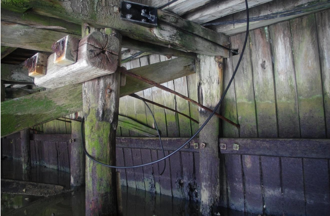
Figure 77: No.3 wharf, typical arrangement of anchor strut and tie rods. Original below with modern repair above
