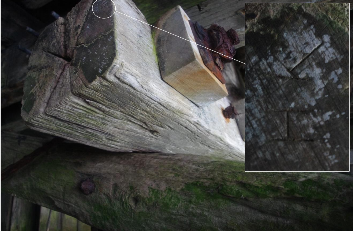
Figure 79: No.3 wharf, cutters mark HK on anchor strut (15.07.2021)
