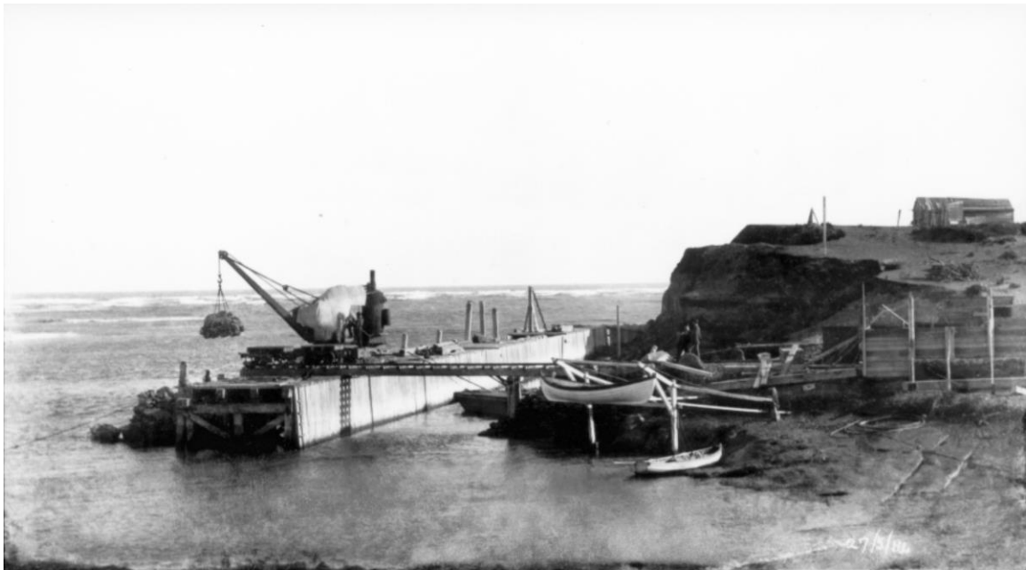
Figure 19: Heads wharf being constructed in May 1884 (Harding & Denton Collection, Wanganui District Library, NZC2.1.271)
