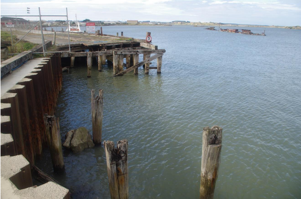
Figure 52: Sheet piling repair to No.1 wharf, with No.2 wharf extending to the east, Te Anau hulk in background.
