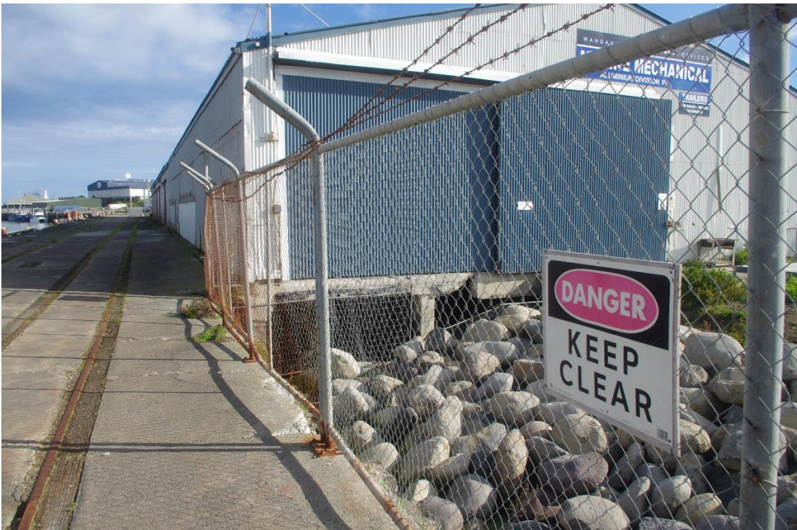
Figure 90: No.3 wharf and scouring beneath Victory shed backfilled with rounded boulders (15.07.2021)
