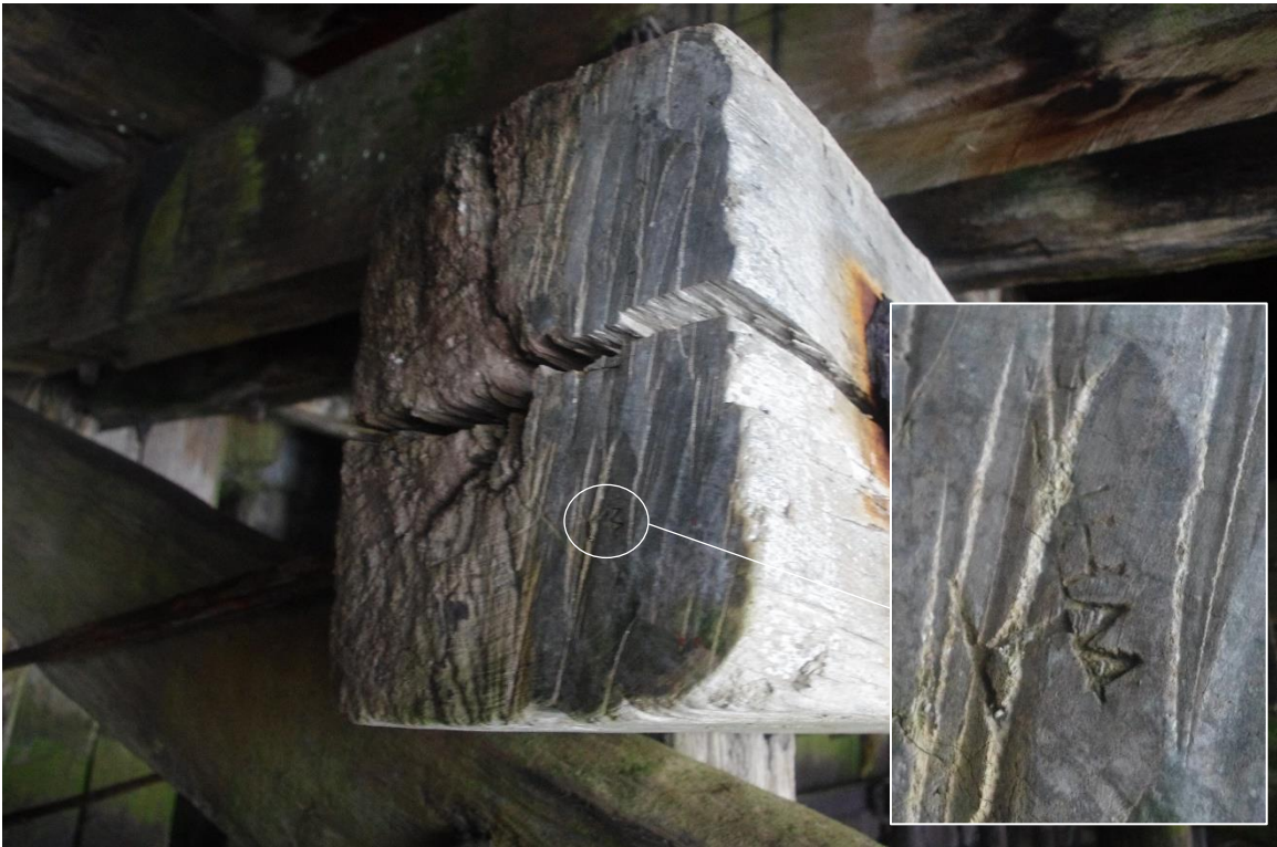
Figure 80: No.3 wharf, cutters mark T WHITE on anchor strut (15.07.2021)
