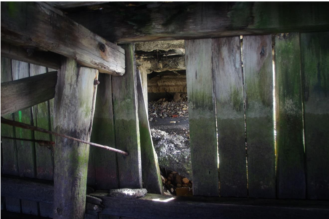
Figure 88: No.3 wharf, eastern end, scoured out fill from behind sheet wall (15.07.2021)
