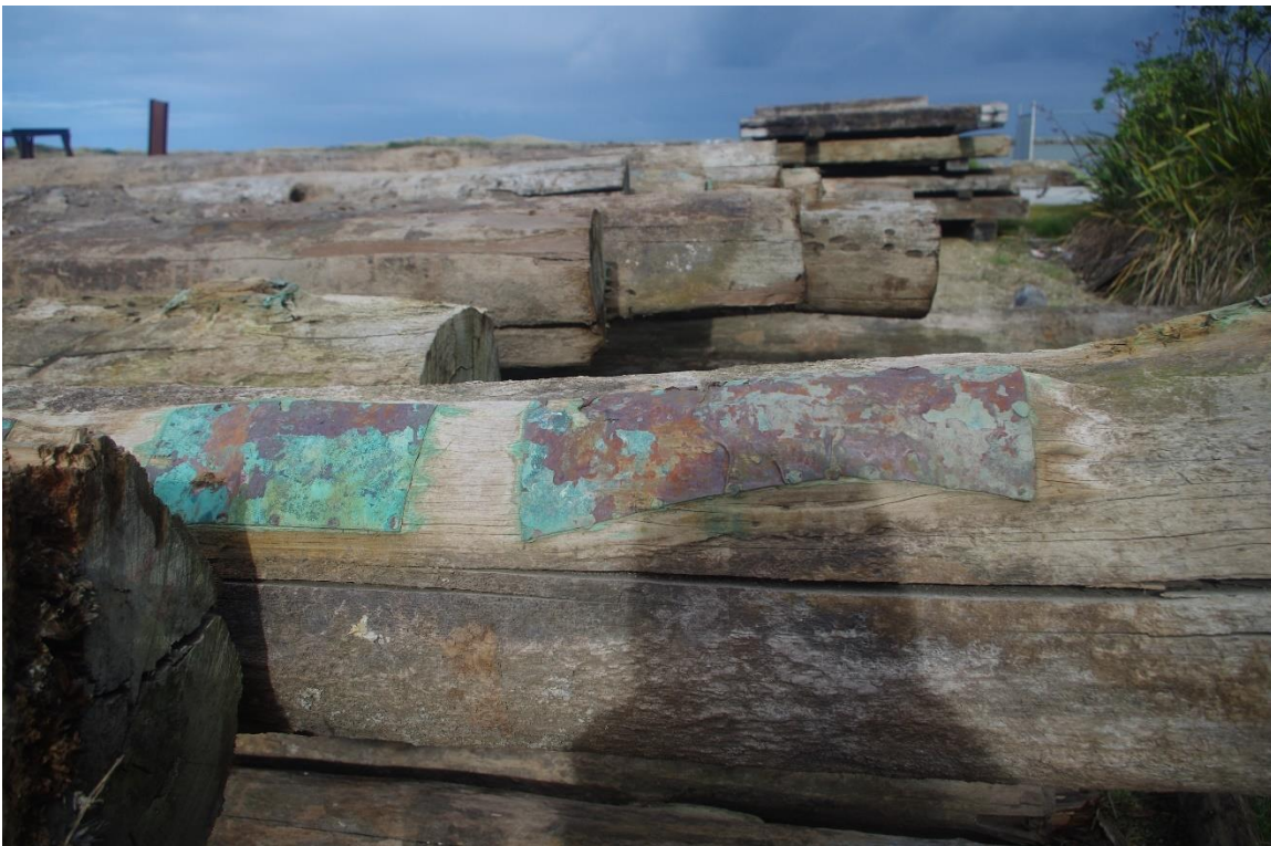
Figure 56: Stock pile. Copper patches over exposed grain or knots on wharf piles (15.07.2021)
