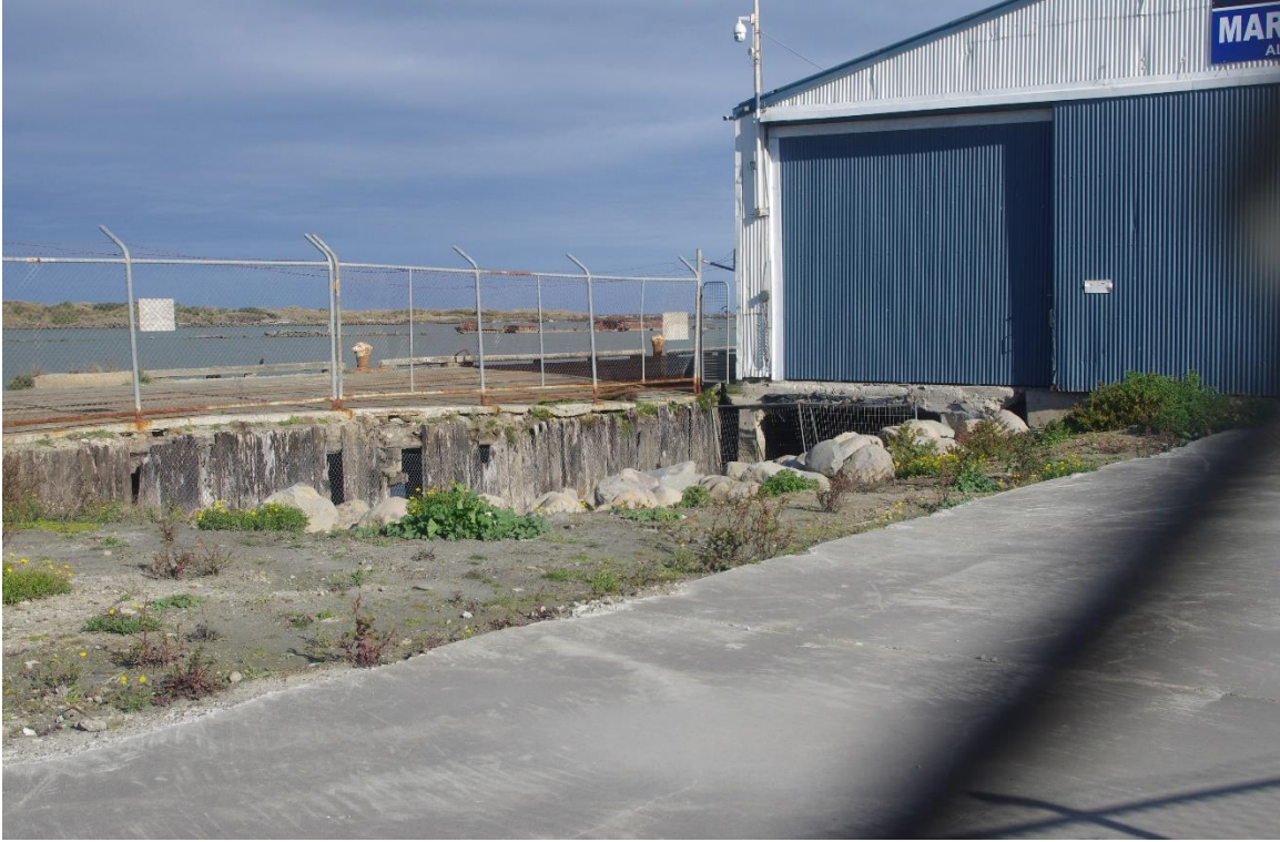
Figure 91: No.3 wharf and scouring beneath Victory shed (15.07.2021)
